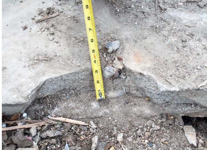
Figure 2.2 Example of catastrophic side concrete breakout at St. John’s Lutheran Church in Pilger, NE
